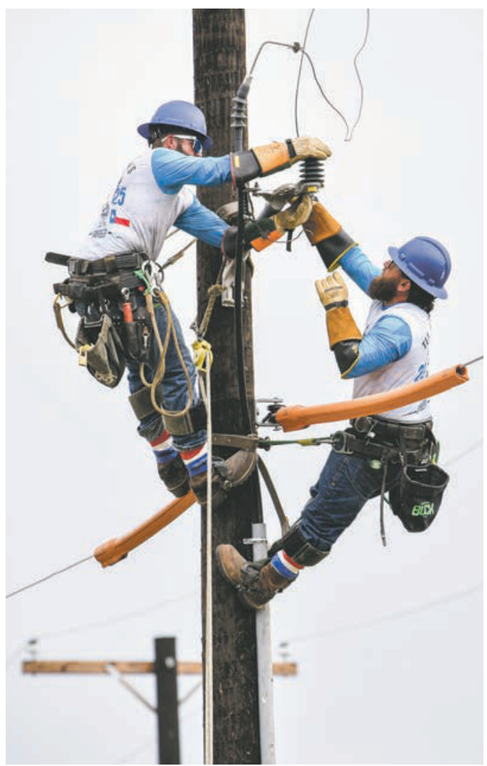
Journeymen Ty Duesterheft and John Zamora from Maxwell change out power line equipment during the 2025 Texas Lineman's Rodeo.
